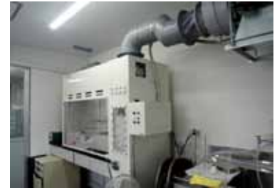
Chemical processing room draft chamber
